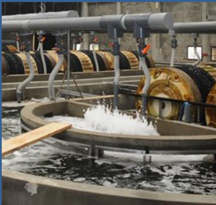
Two SAFF-38Lps multiple-tube airlift water pumps installed in a marine RAS producing Gilthead sea bream ( Sparus aurata ) in Tartous, Syria.
