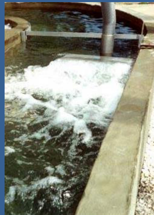
The SAFF-120 (MK1) medium-bubble airlift aerator operational at the Hadath Tilapia Farm, Lebanon (year 2000) and a side elevation of the aerator.
